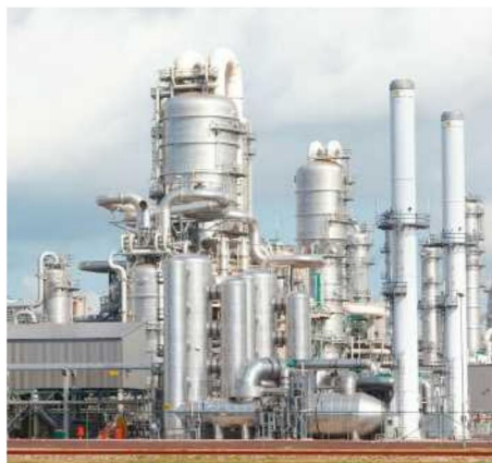
System expansion and post installation
